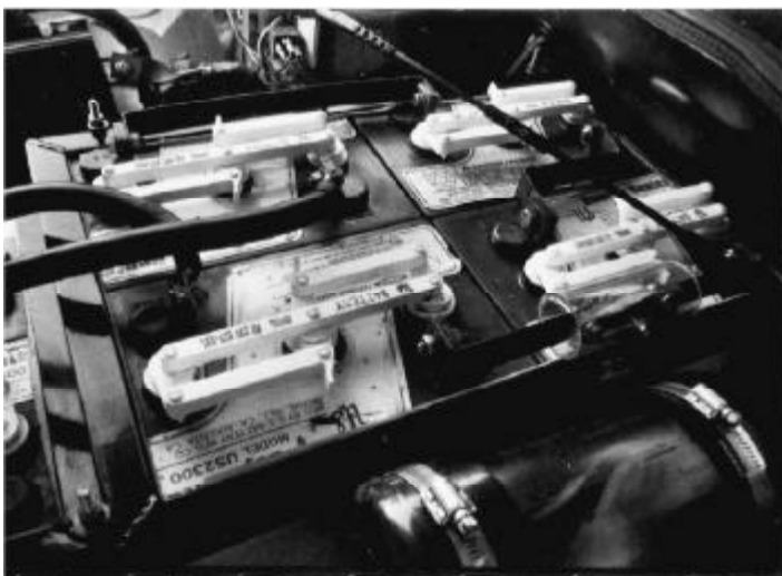
Copper straps between batteries, and cables connecting to the lower level of the pack.
