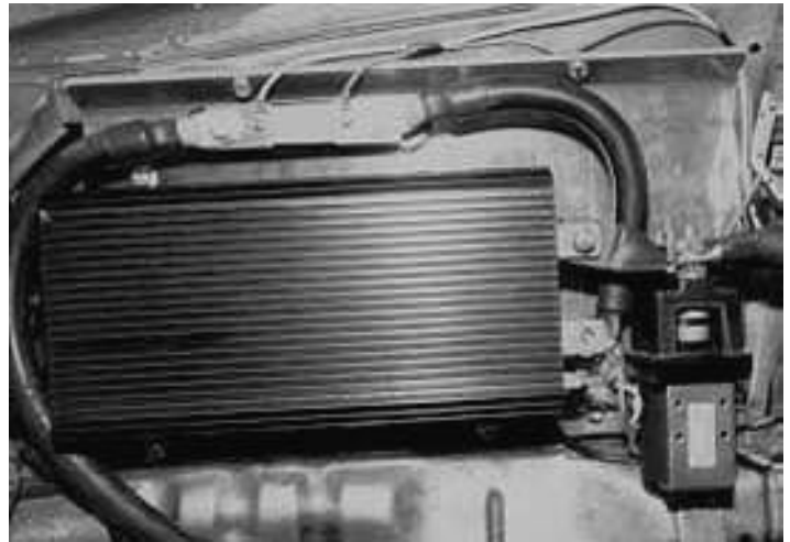
installed ontroller, contactor, shunt
